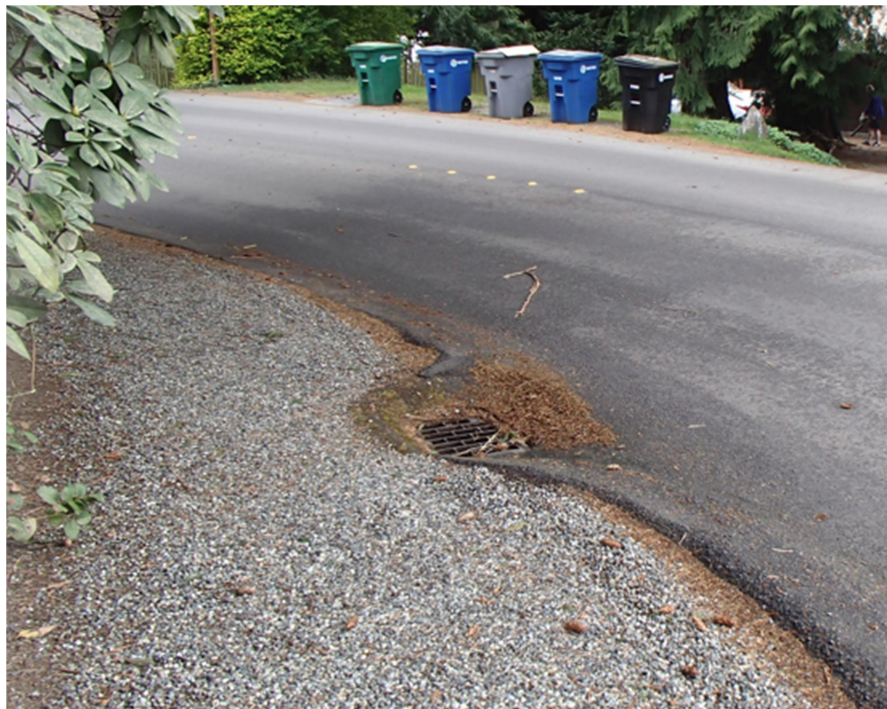
Photo No. 8 Looking southerly at CB #30a-51 opposite House #6035. Note accumulation of fir needles, but still appears to be draining well.
